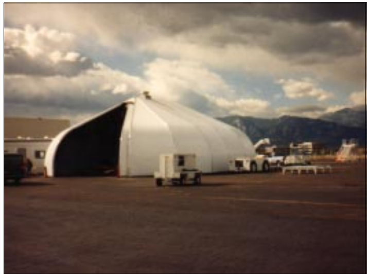
Chance screw anchors helped speed up the construction of this temporary storage building.
