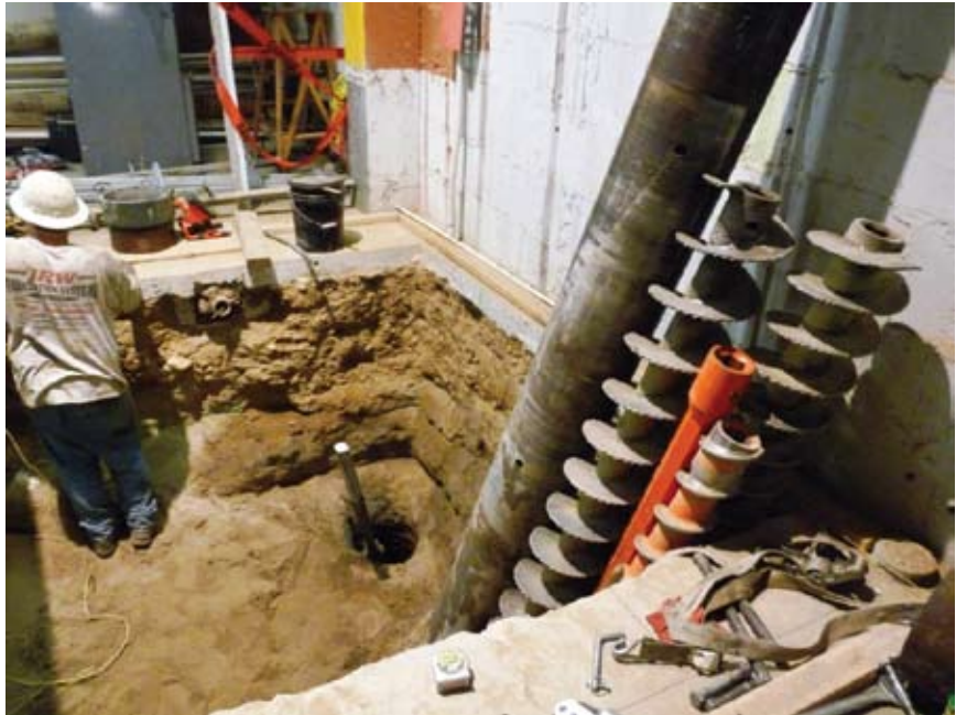
Chance® Micropile installed in tight working conditions on this job. Note custom-designed continuous-flight auger and casing at right.
