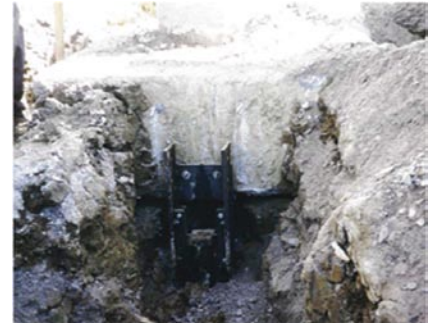
Success: Pier configuration after installation and restoration of the structure. Notice void below the footing indicating the 2-3/4 inch lift of the footing and structure.
