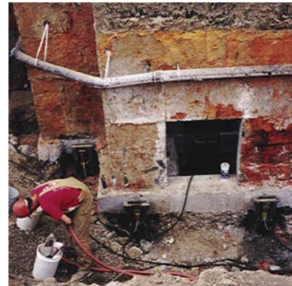
Photographs at right show how the Atlas Resistance® Piers were installed inside of the window well. In order to gain access to the footing, the gravel fill at the window well was removed. Access holes were cut through the wall at the window well to gain access as shown in the lower right photograph.
